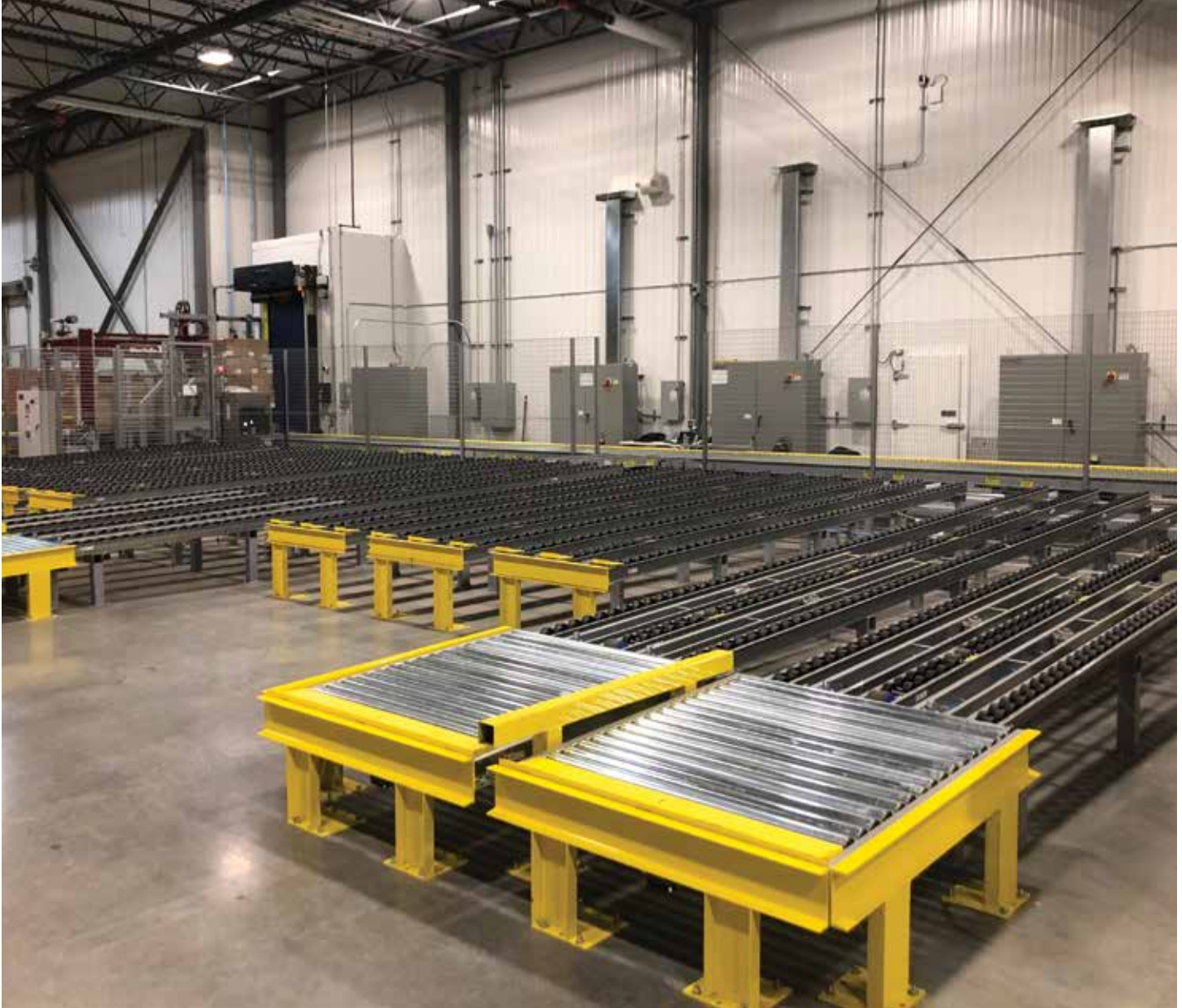
There is a pinwheel design on both inbound and outbound conveyance, which allows for efficient pallet handling in the loading and unloading processes. (Photo courtesy of UISC.)
