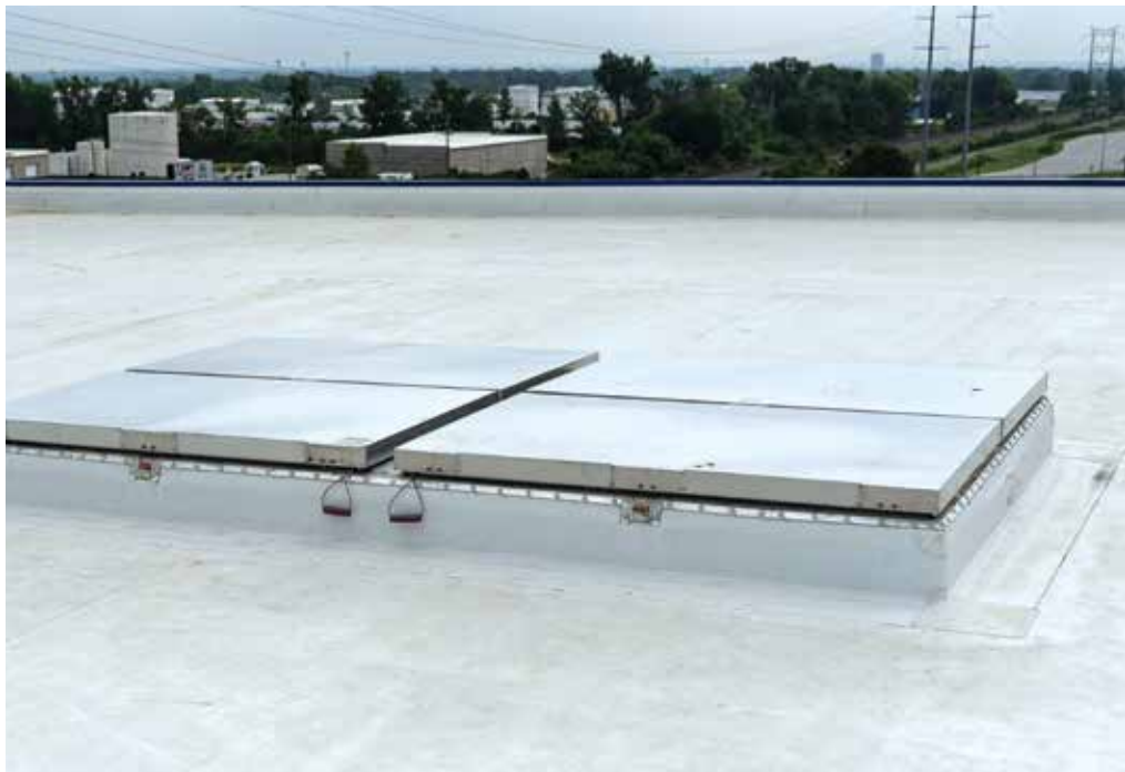
Custom-made smoke vents enable firefighters to enter the building safely to better control a fire. (Photo courtesy of Dick Cold Storage.)
