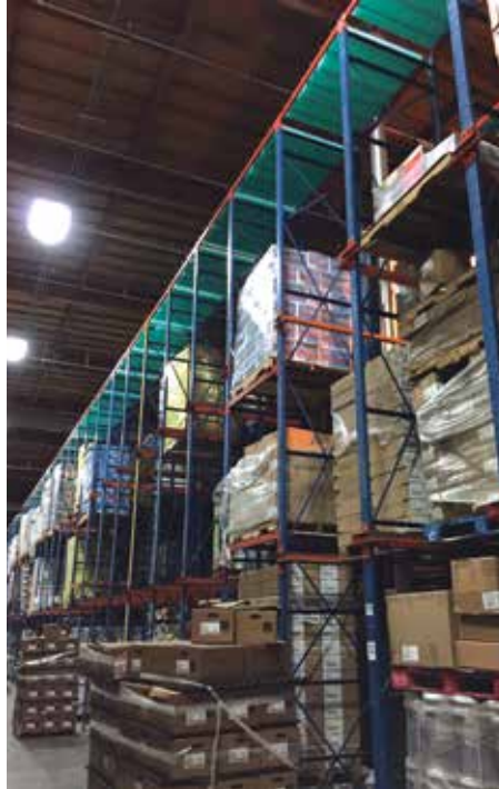
Thermal Energy Storage modules installed on top crossmember of the racking structure. (Photo courtesy of Viking Cold.)
