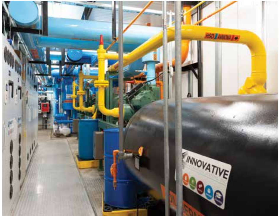
Energy efficient measures were incorporated in the refrigeration system including VFDs, energy efficient motors and an ammonia central system. (Photo credit Curtis Waltz, Aerialscapes. Photo courtesy of ESI Group USA.)
