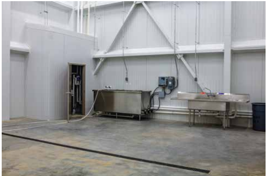
ARCO provided a turnkey project for MTC Logistics in its new poultry distribution center. (Photo courtesy of ARCO Design/Build.)
