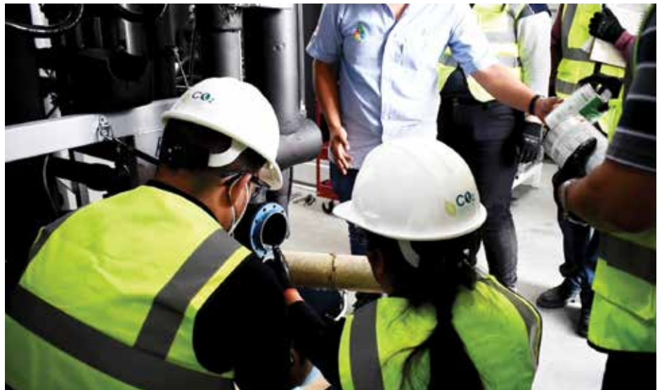
Technicians and engineers carry out maintenance practices on a CO 2 system already in operation in the machine room in Mexideli's new distribution center in Mexico City, Mexico. The training was carried out by the CO 2 Training Center Mexico and SRT team members. (Photo courtesy of Sistemas de Refrigeración Totales.)
