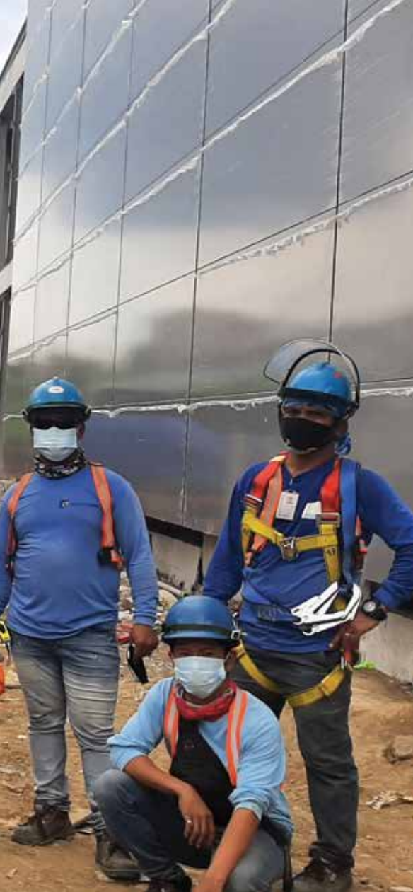
Construction sites in Asia began to reopen in early June. (Photo courtesy of CT-Technologies.)
