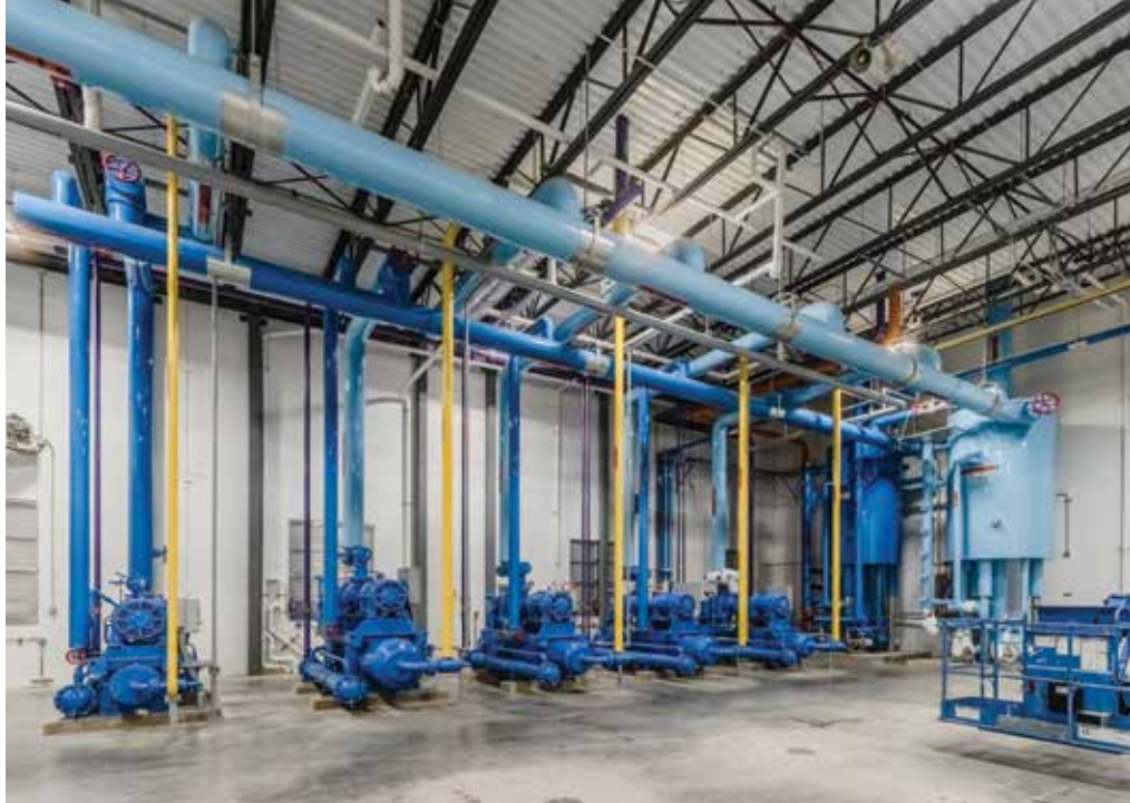
The plumbing and electrical in the engine room was encased in flowable grout instead of concrete to save time. (Photo courtesy of Primus Builders, Inc.)
