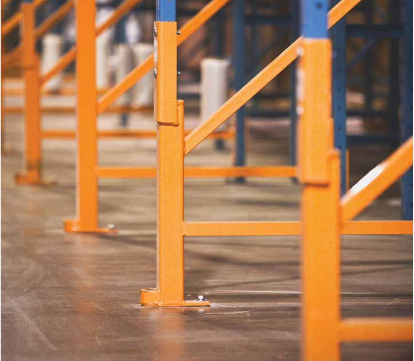
Rack repairs should be done by crews that are familiar with installing rack repair solutions. (Photo courtesy of Damotech.)
