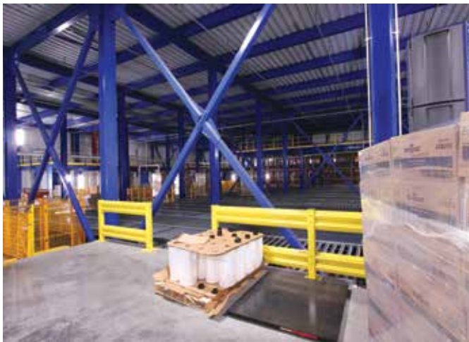
Uninterrupted pallet racking with unobstructed areas within can reach 135 feet. (Photo courtesy of Fisher Construction Group.)
