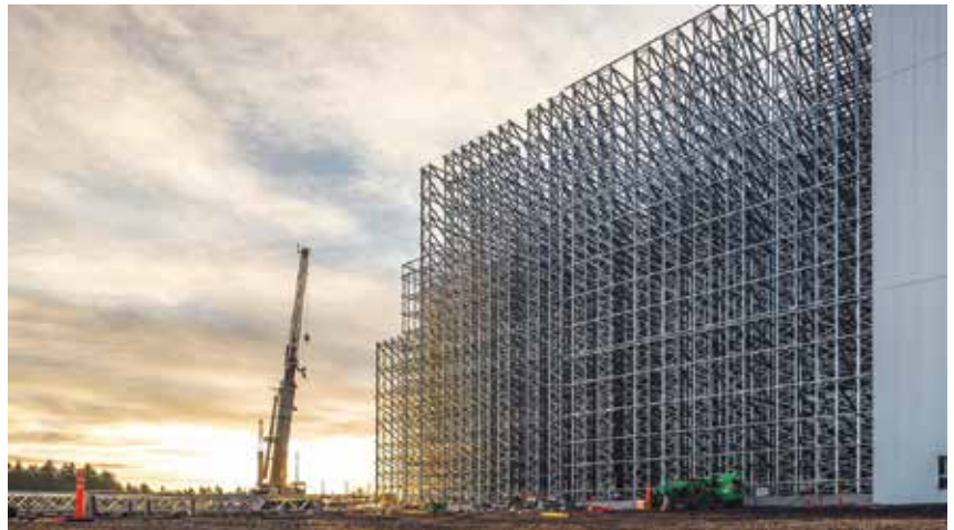
The NewCold Tacoma state-of-the-art freezer is a joint design effort by Netherlands-based NewCold Advanced Cold Logistics and the design/build firm Fisher Construction Group of Burlington, Washington. It is one of the largest cold storage facilities in the United States, with Phase 1 containing approximately 25 million cubic feet of storage capacity an 103,000 pallet positions. ((Photo courtesy of NewCold.)
