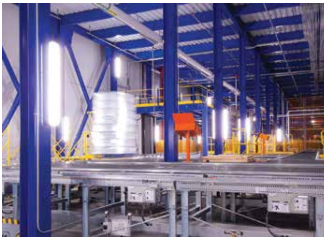
A section of the 1.5 miles of conveyors contained within NewCold Tacoma. (Photo courtesy of Fisher Construction Group.)
