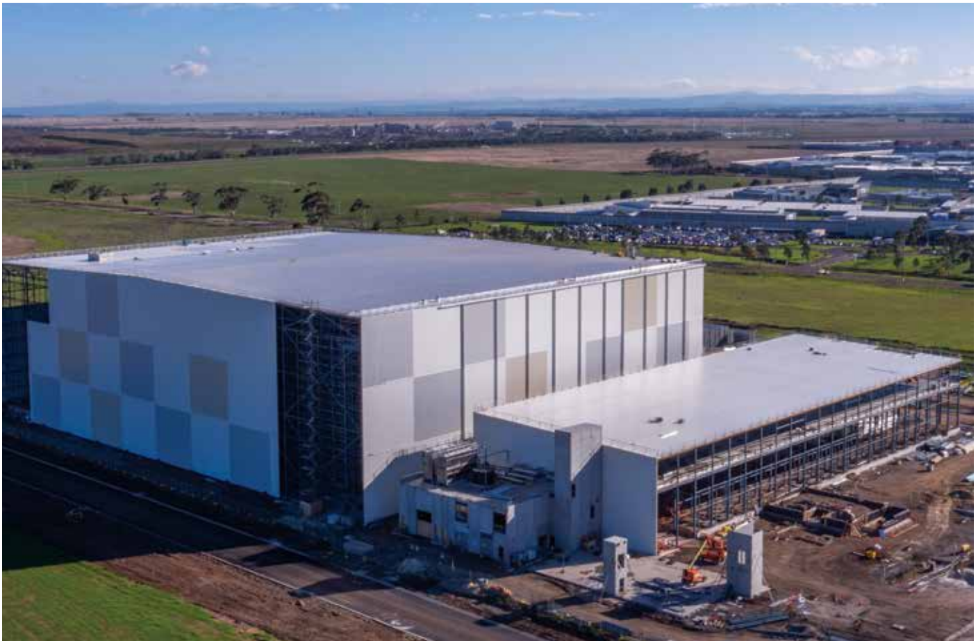
Constructed by NewCold in Melbourne, Australia, with the insulated envelope and specialty doors contributed by ISD Solutions, this is the first fully automated high bay cold storage facility on the continent and the largest in the Southern Hemisphere with the capacity of 100,000 pallet spaces and measuring approximately 135m x 105m x 36m high. (Photo courtesy of ISD Solutions.)
