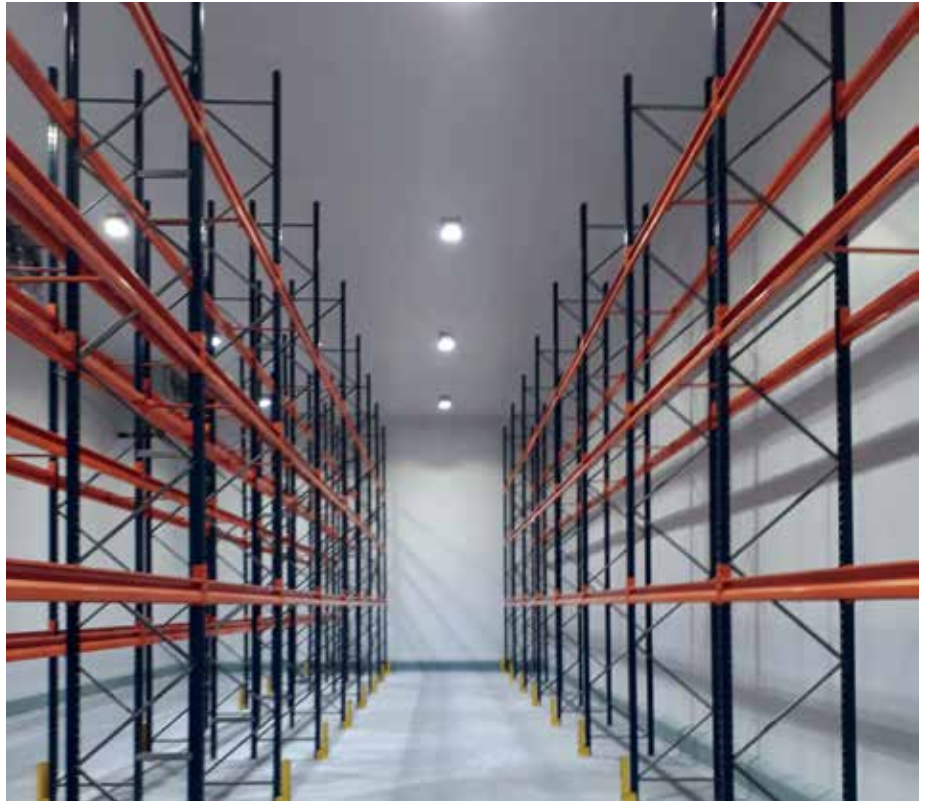
A refrigerated warehouse for fish production and storage built by Civil-Frio in Rio De Janeiro. (Photo courtesy of Civil-Frio.)
