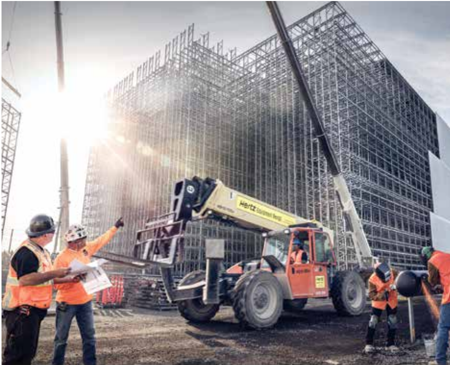
SubZero Refrigeration Superintendent talking with his team about rigging mechanical equipment at the 120-foot elevation. (Photo courtesy of SubZero Constructors.)
