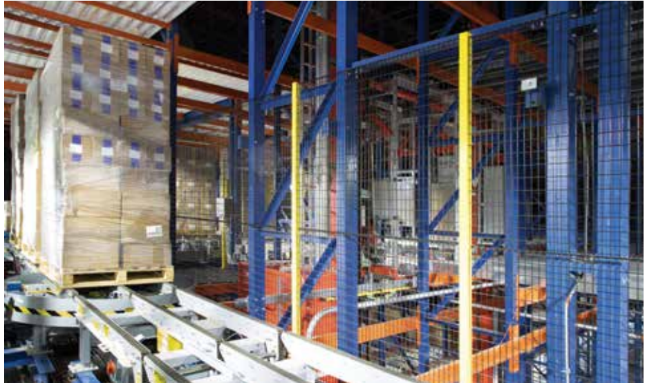
From truck to freezer, automated conveyors carry product throughout the conveyor tracks. (Photo courtesy of Fisher Construction Group.)
