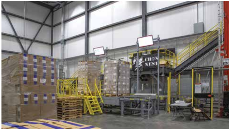
The conveyers are operated from a crow nest that can regulate product flow between the loading dock and freezers. (Photo courtesy of Fisher Construction Group.)
